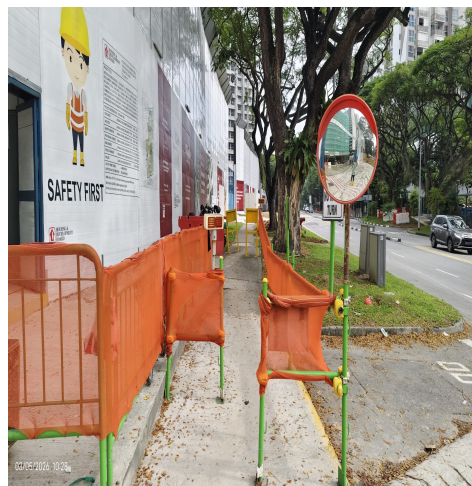
Excess GI pipe as barriers
